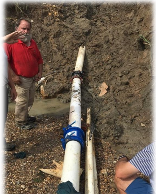
Figure 2-3. Fixing a leaking irrigation pipe at Tavern Creek Golf Course (St. Albans, MO).
