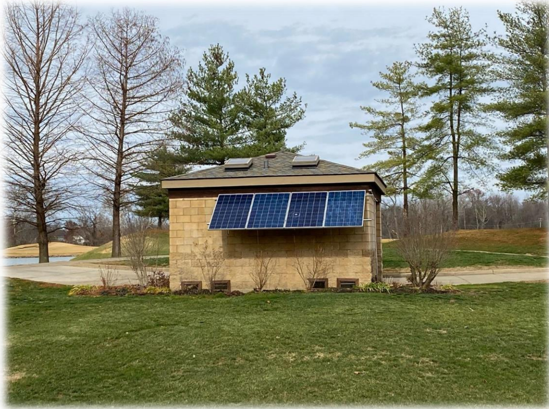
Figure 13-1. Solar panel used to power water and ice machine at Old Hickory Golf Club (St. Peter's, MO).
