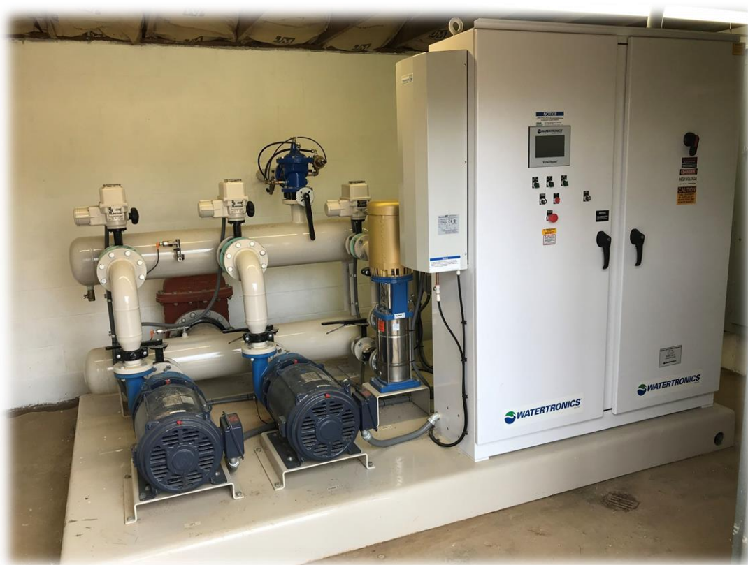
Figure 2-2. Gravity fed horizontal end suction pump system with VFD control panel at Bogey Hills Country Club (St. Charles, MO).
